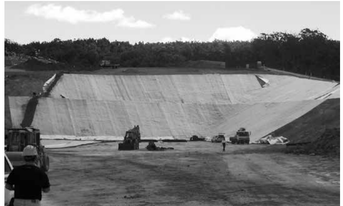
Figure 1. Geosynthetic Clay Liner (GCL) being used to line a landfill site. The bentonite within the GCL has to meet various specifications such as particle size, swelling characteristics, fluid loss and permeability. Source: AMCOL Australia.
